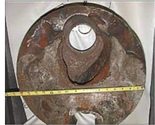
Corrosion of Davis-Besse reactor vessel head [1]
