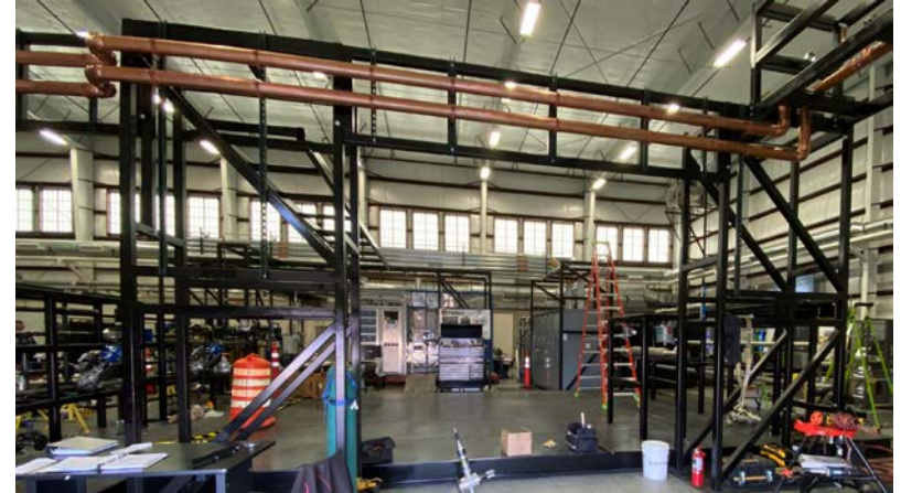
MAGNET Skid and Pipe Racks
