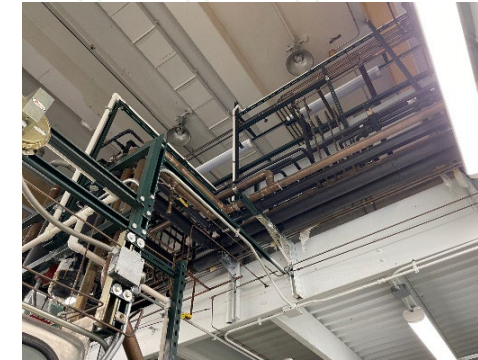
Mezzanine-level cooling jackets
