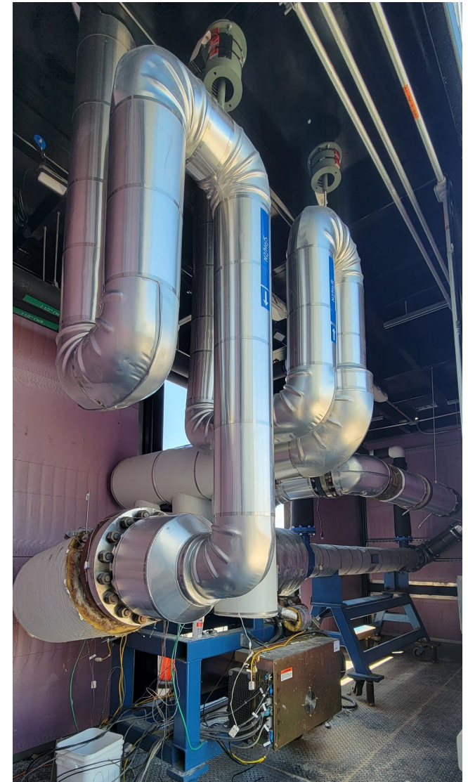
Portion of Added Piping
