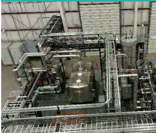
Helium Component Test Facility [2022]
