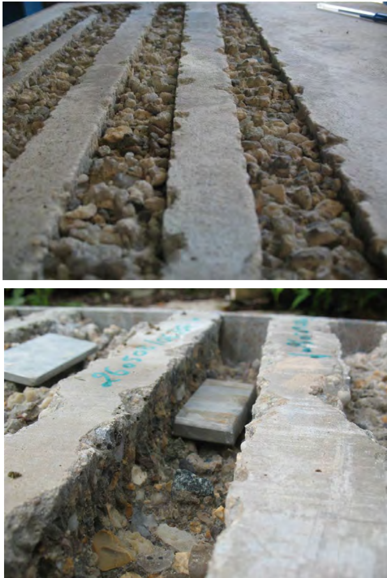
Figure C-1: Concrete Scabbled via NitroJet®: (Top) without Aggregate Removed and (Bottom) with Aggregate Removed [1]
