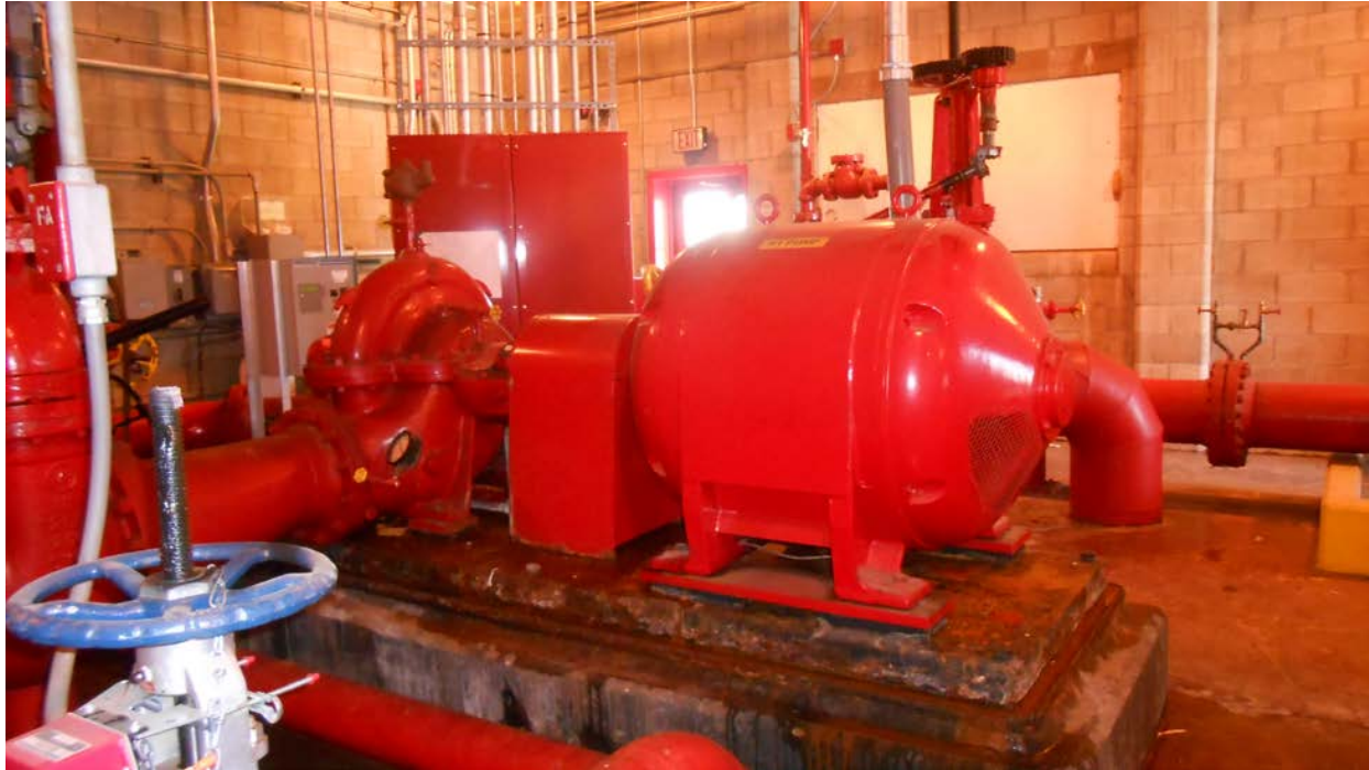
Figure 4-3: HPFW System Pump House
