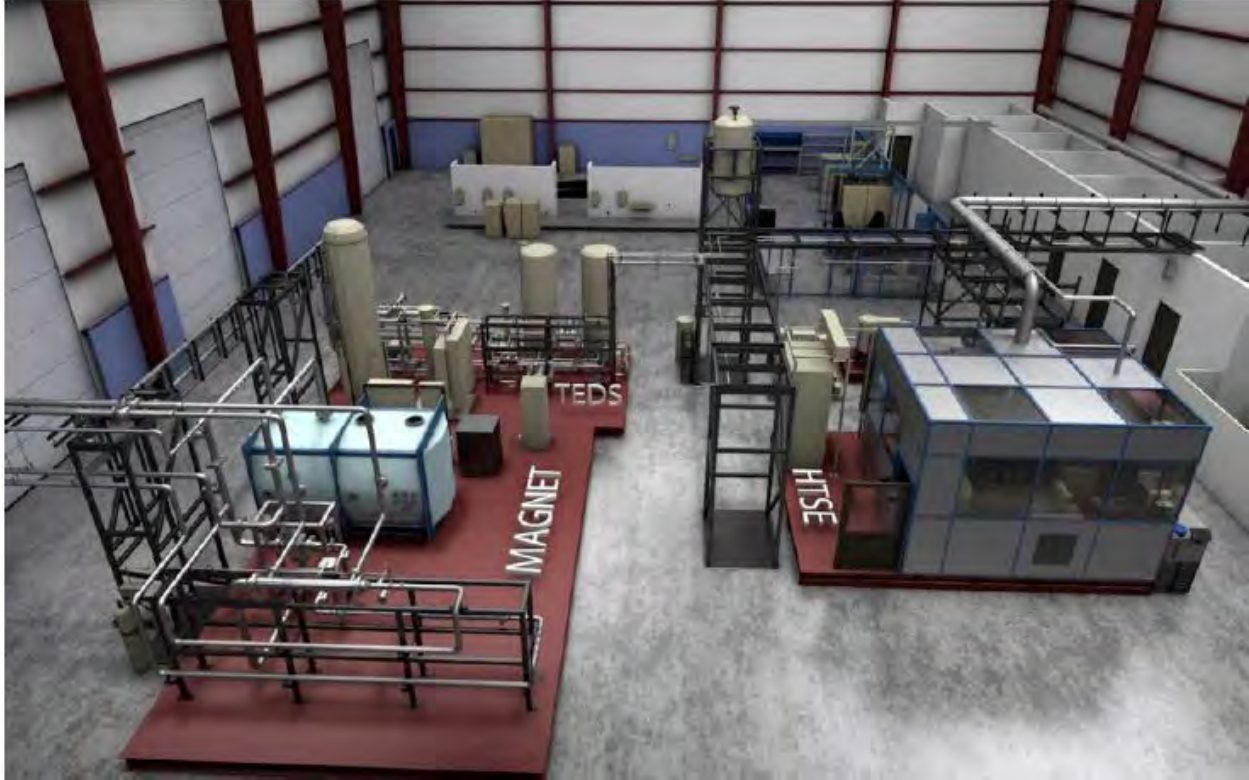
Figure 1. MAGNET deployment in INL's Energy Systems Laboratory building, Systems Integration Laboratory.
