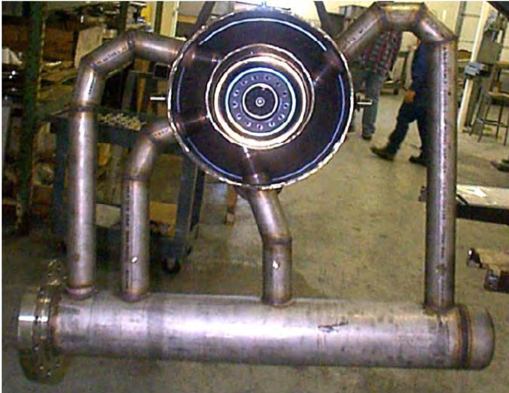
Figure 10. Photograph of Capstone C30 piping modifications to divert the recuperator cold-side outlet stream to external heater unit.
