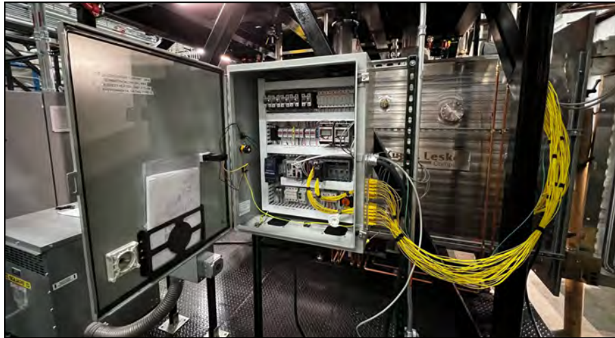
UW control panel
