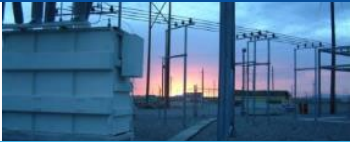
Commercial Feeds, Test Loops/Spurs
