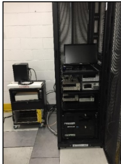
Experiment DAS cabinet to support instrument testing at the TREAT facility
